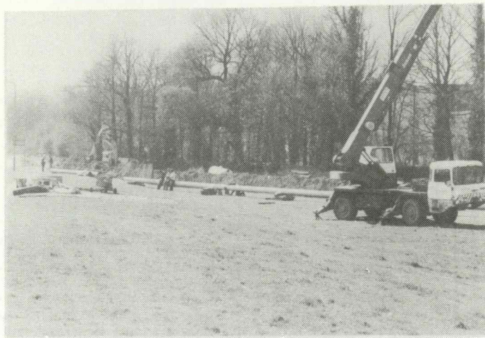
The A27 frontage of the University has recently been the scene of major excavations while the national gas network main has been realigned.
