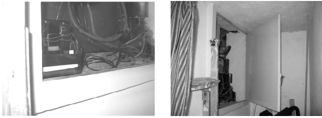
Fig. 3 Left. Sensor in the corner of the mains cabinet, Right. The mains cabinet to the house by the ceiling of the corridor.
